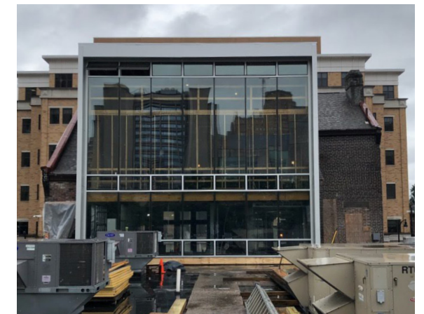
View from existing north roof toward new curtain wall during glazing installation.
